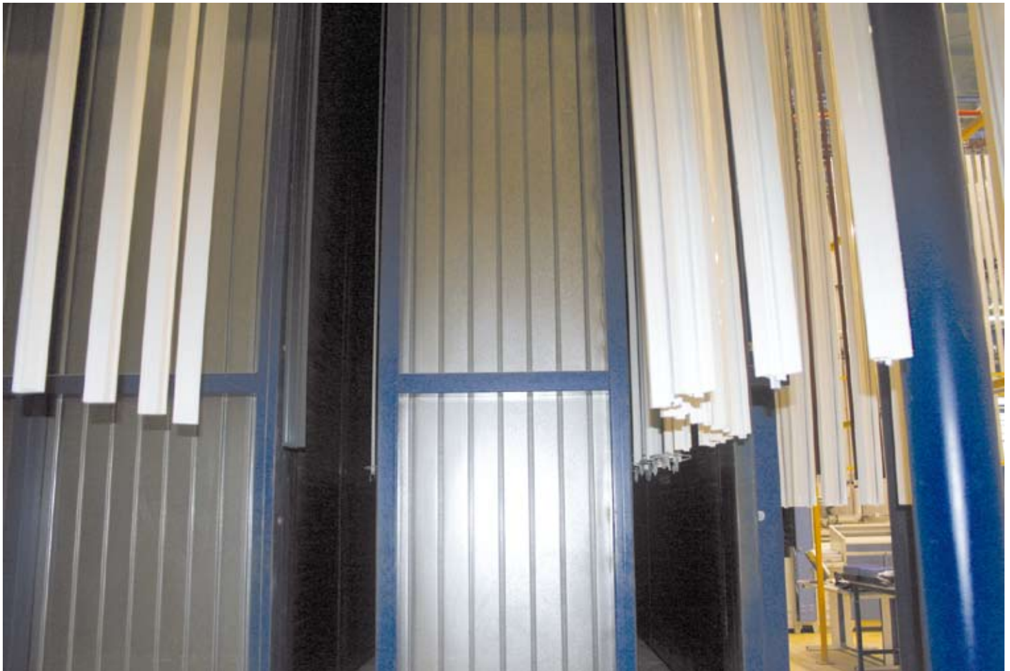
17 - The entrance and exit of the infrared polymerisation oven.
